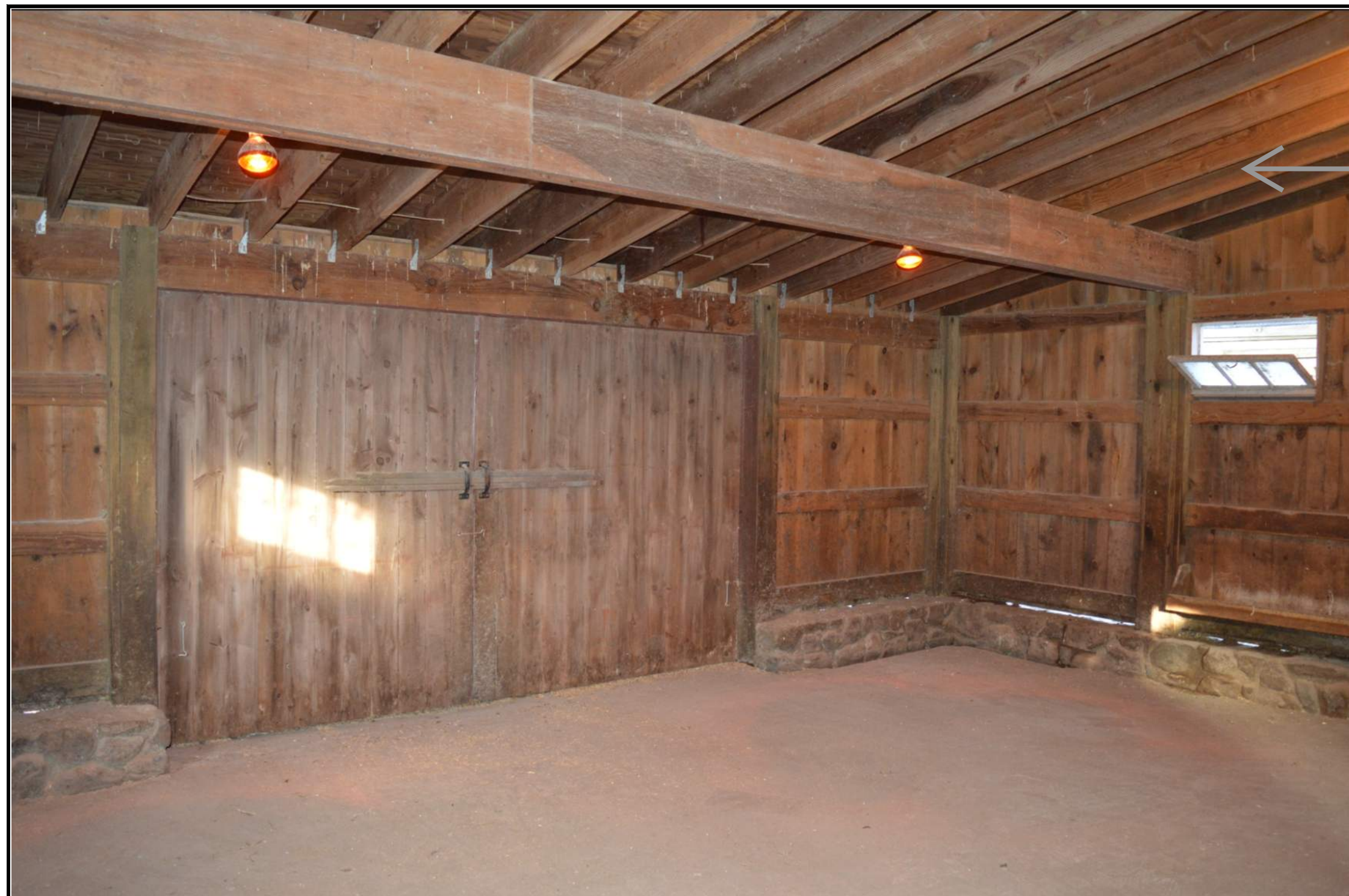
Roof made of modern lumber, rafter clips, and hangers. Not original to barns.
