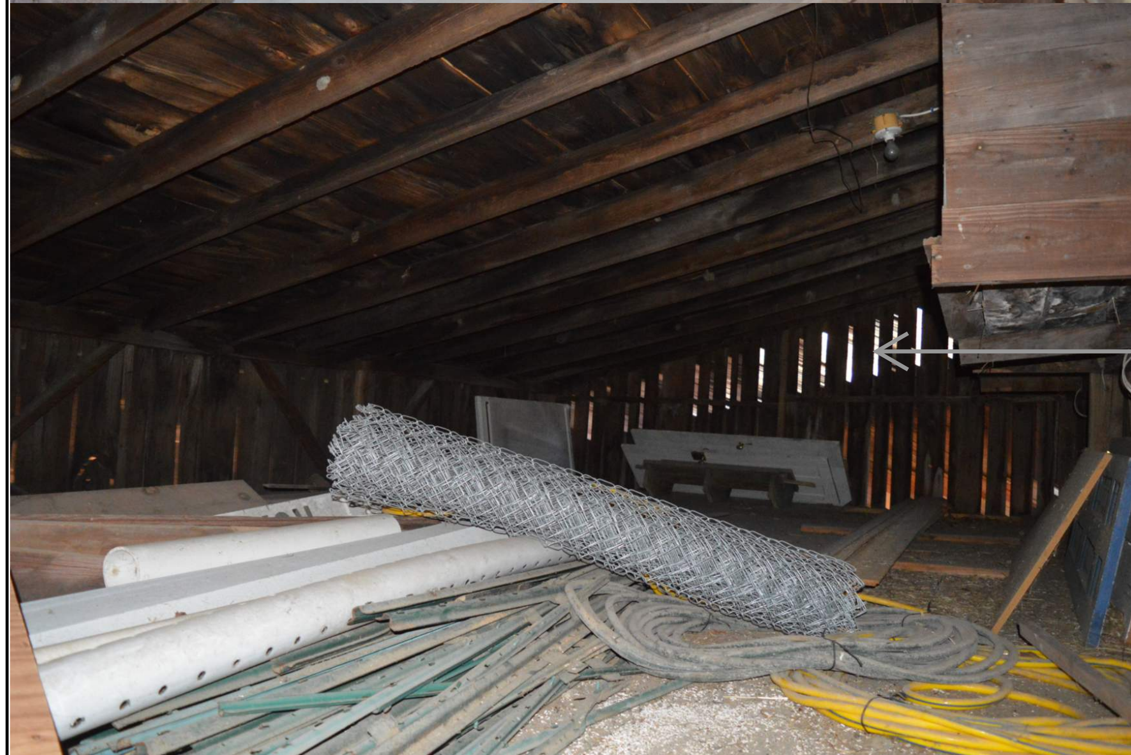
Large gaps in wall material allowed in weather and deteriorated materials
