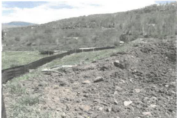
A topsoil stockpile that has been partially revegetated and is protected by silt fence perimeter control.
